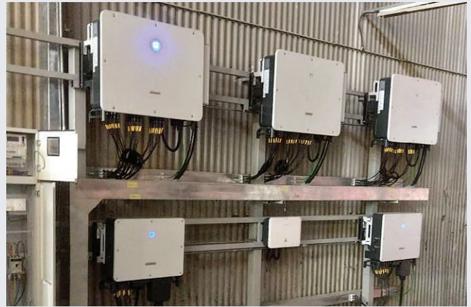
Figure 4: Meter and Breaker Panel, and Inverter Station at KHCS Plant 2
