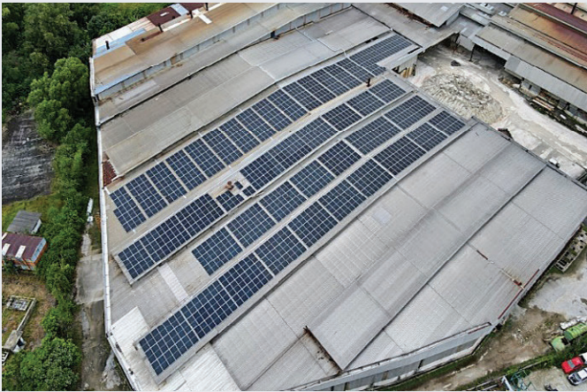
Figure 3: Rooftop solar PV system installed at KHCS Plant 2
