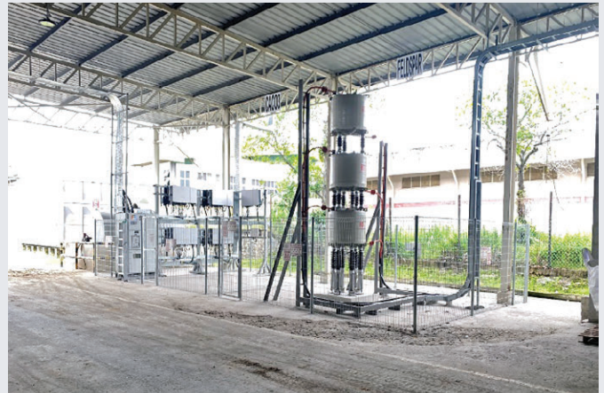
Figure 2: Meter and Breaker Panel, Inverter Station and Fault Current Limiting Reactor (FCLR) at KHCS Plant 1
